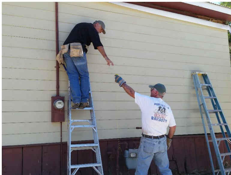
Teamwork in action...Art Long (right) hands Alan Roberts a chalk line as the two Rotarian volunteers complete the remodel of the ACHS mine model.
