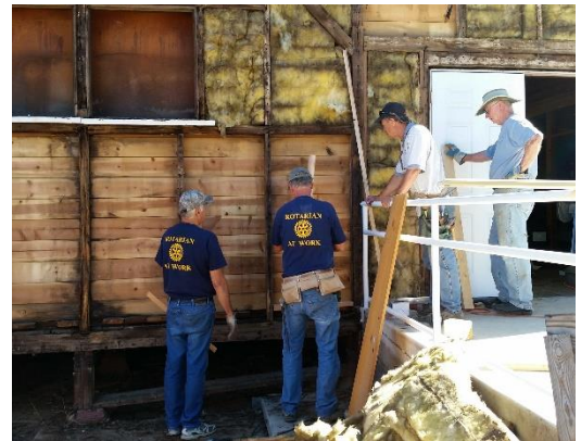
Rotarian crew members, (left to right) Keith Sweet , Alan Roberts , Phil Giurlani , and Art Long confer on installation of new siding on the Mine Model housing.
