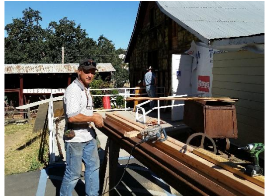
Phil Giurlani tackles the task of replacing siding on the Mine Model Building.
